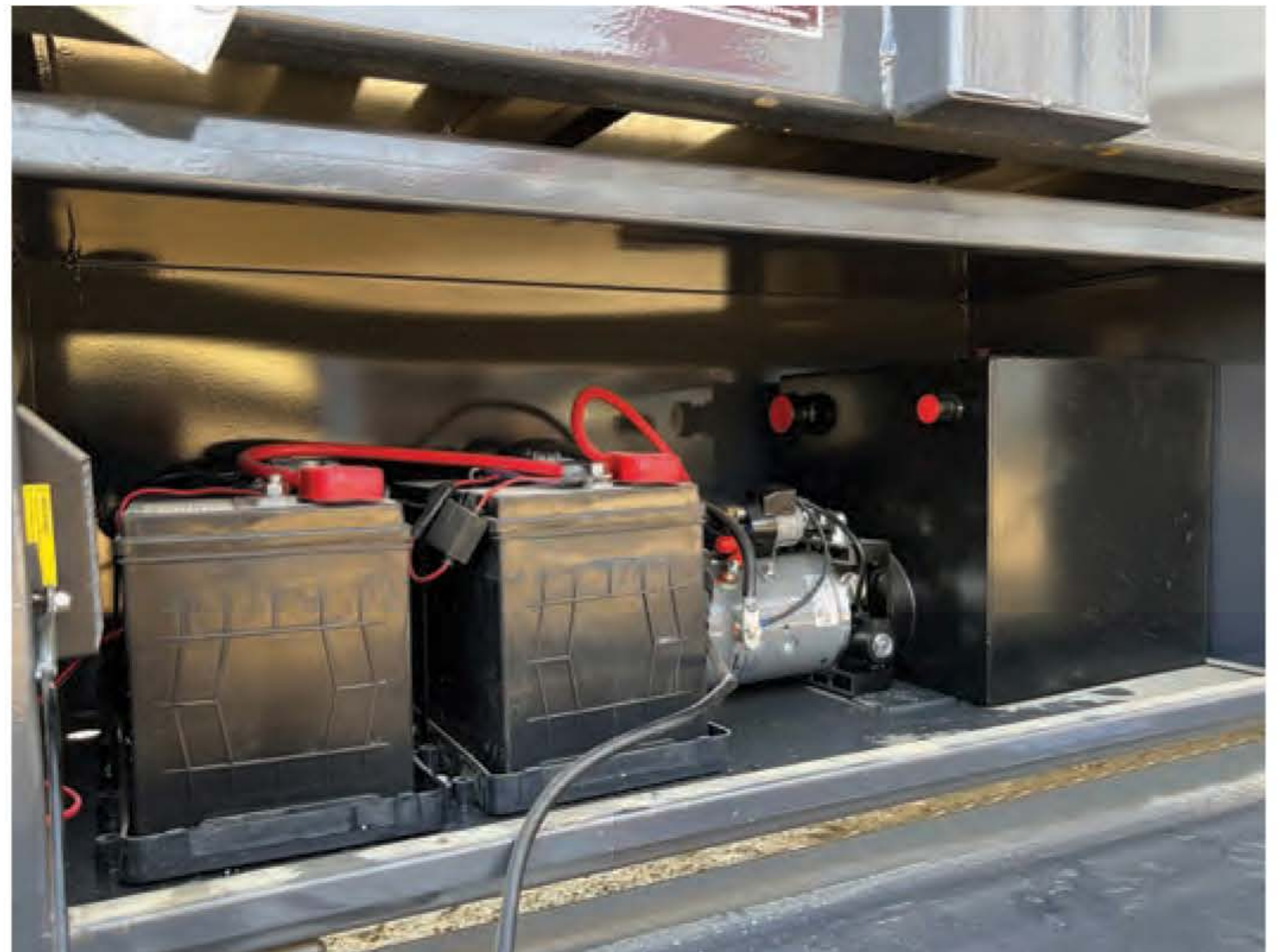
Locking Battery & Pump Box
